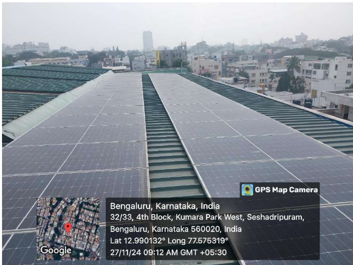
Solar Panels at Seshadripuram Institute of Commerce and Management
