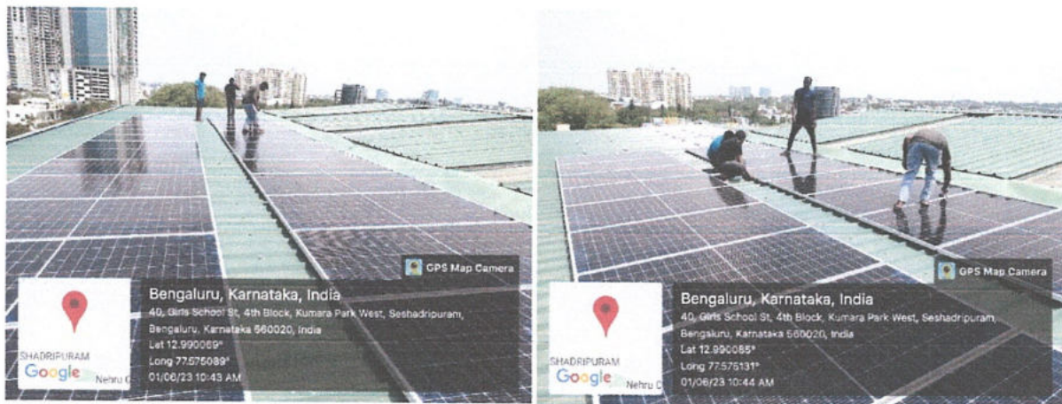
Figure 4: Solar Panels at Seshadripuram Institute of Commerce and Management
