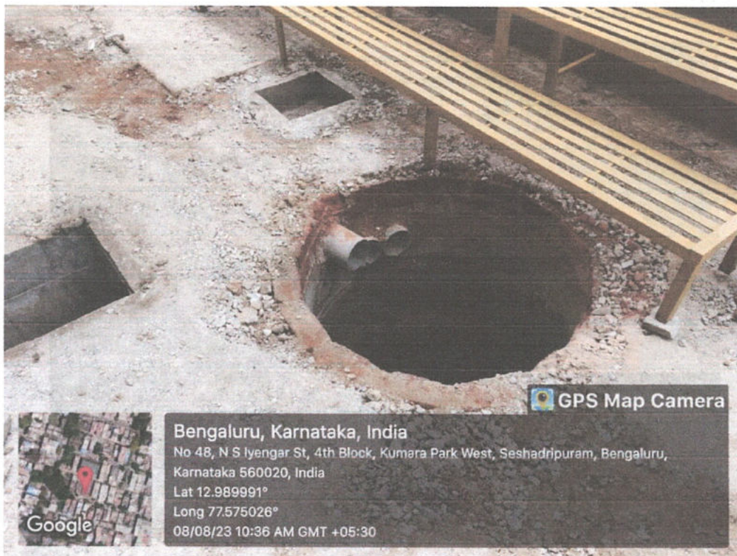
Figure 6: Rainwater recharge pit
